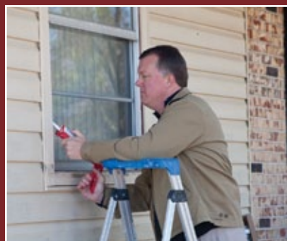
WINDOWS Remove dried out molding and replace with fresh caulk
